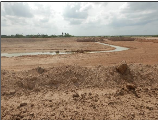
Photograph 8 – View looking west at the location where the existing Raymondville Drain turns west.
