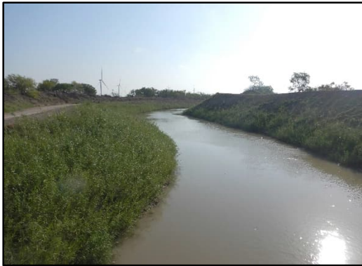
Photograph 103 – View looking east (downstream) at the existing Raymondville Drain. East of this location, most of the RDP study corridor was inaccessible due to a lack of right-of-entry permissions.
